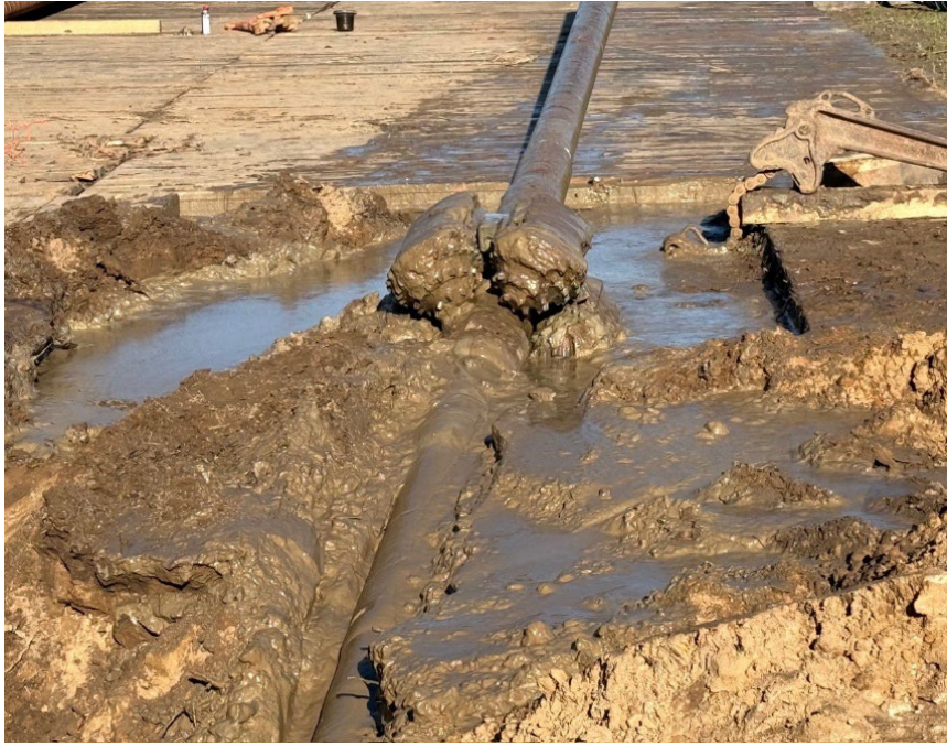
Facing west near MP 3.0, commencing the first ream pass on HDD P4-5
