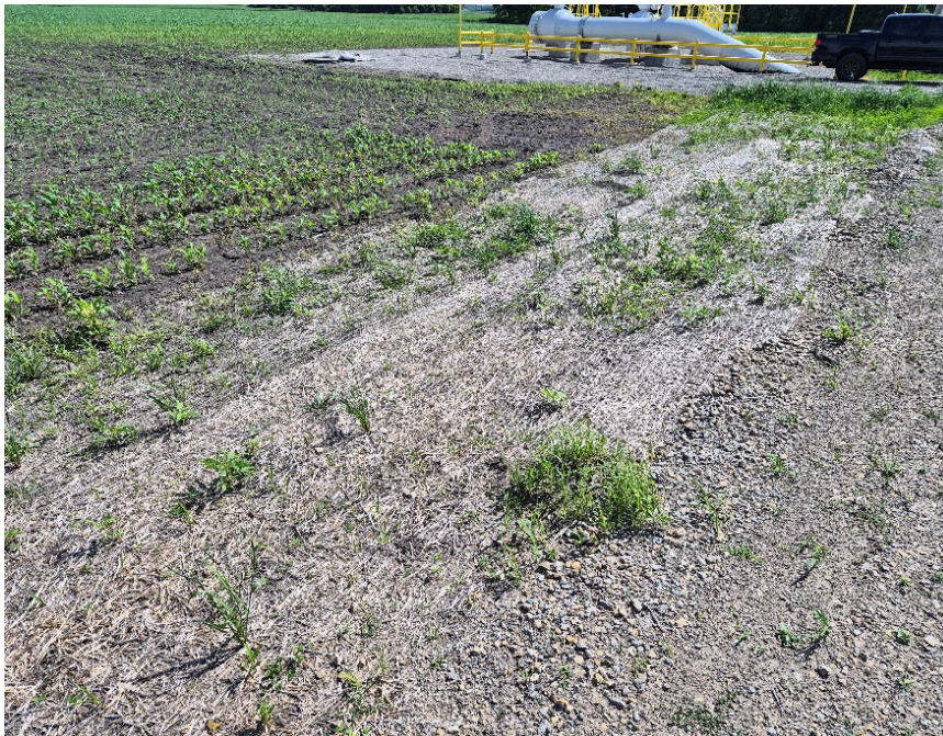
Facing northeast at MP 34.2, ECB functional and ditch at 15 percent of adjacent vegetation
