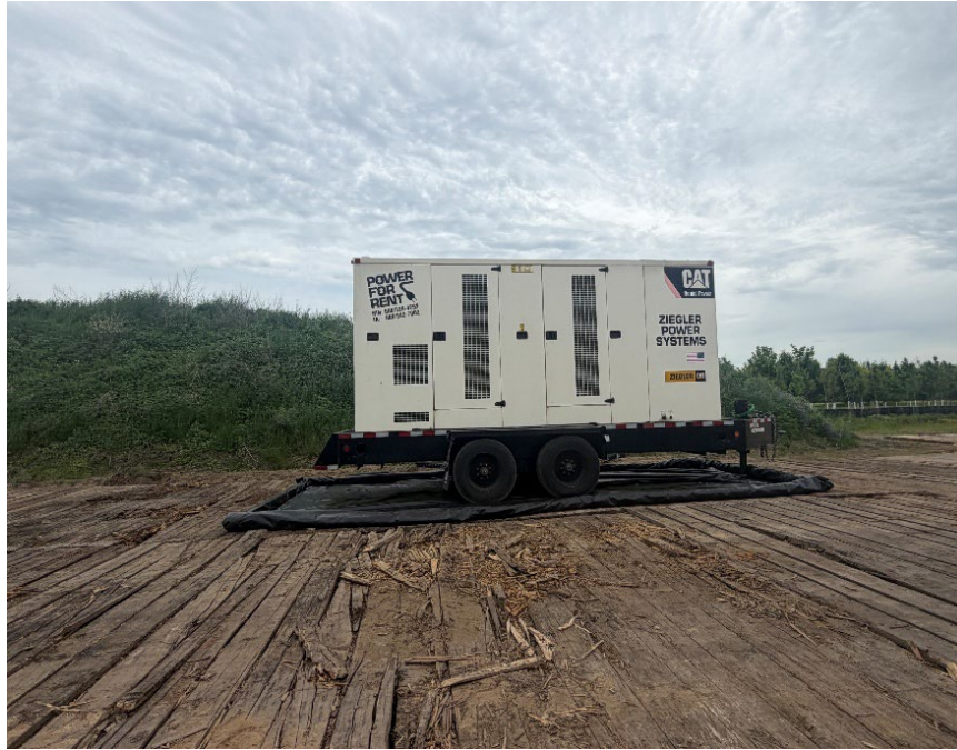
Facing north near MP 3.0, equipment placed in secondary containment
