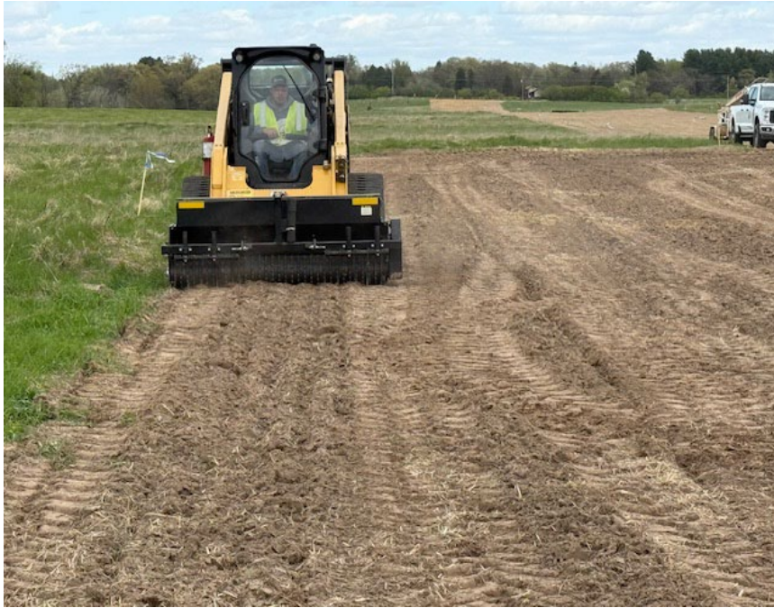
Facing north near MP 1.4, Otis seeding MNL pollinator wet mesic seed mix on the MDNR property, a skid steer was utilized to seed cross slope, where necessary, to reduce rill erosion
